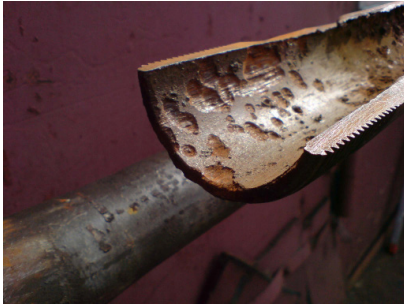
Why did this pipe fail?
