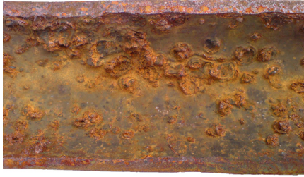
MIC Corrosion Inside Pipe
