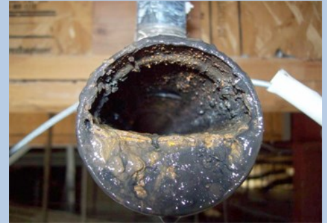
Dry sprinkler system, 5 years old
