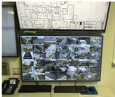
Monitors located in the security guard area show the system being monitored in real time.
