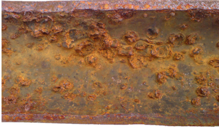
MIC Corrosion Inside Pipe
